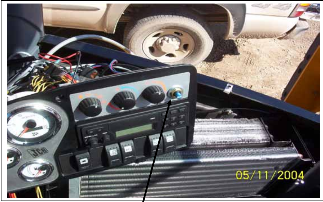
Mount A/C on-off push button switch in existing hole in metal panel behind decal.
